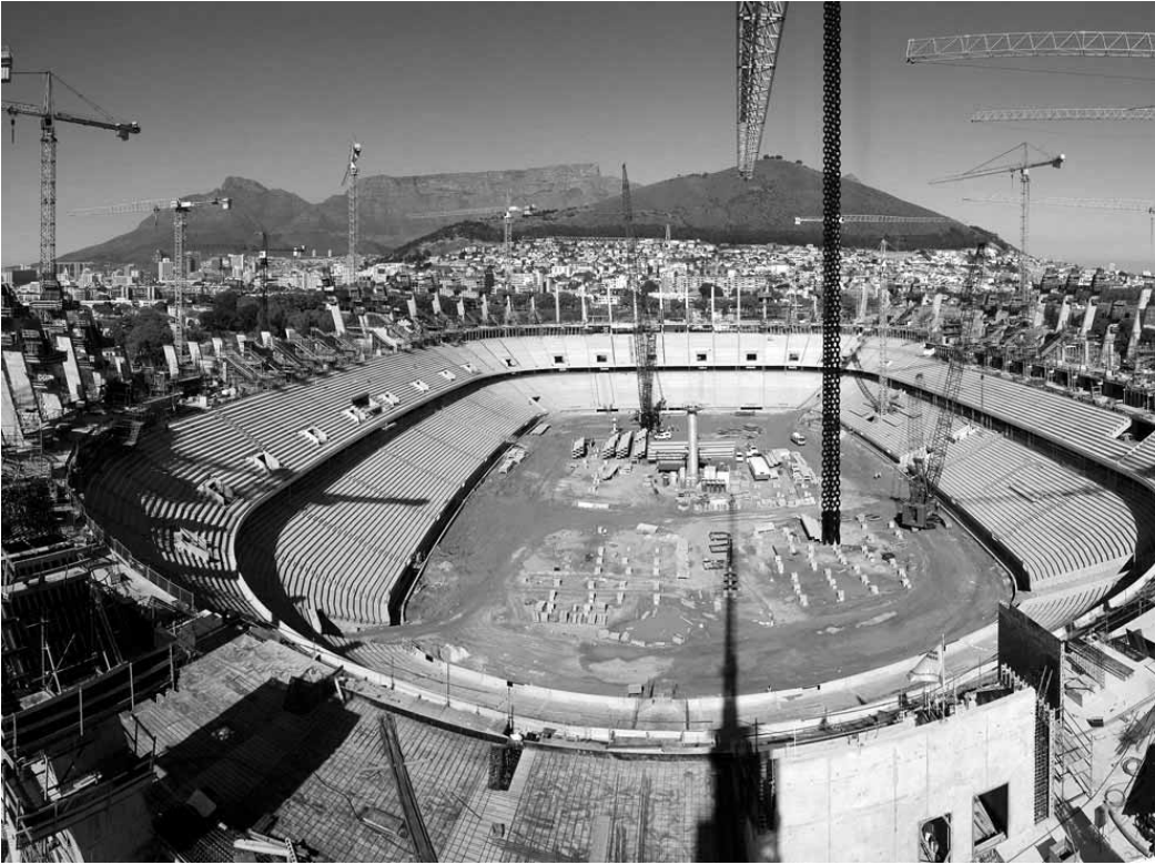
Cape Town's Greenpoint stadium under construction: The state-led infrastructure programme is the one sector that has consistently contributed to growth and employment
